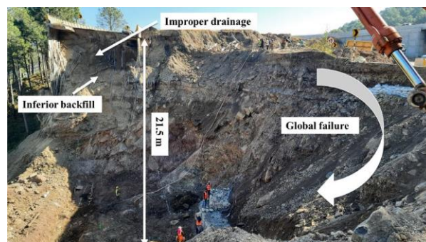
Figure 1. Image of the failure of the wall section after the 2022 monsoon.
